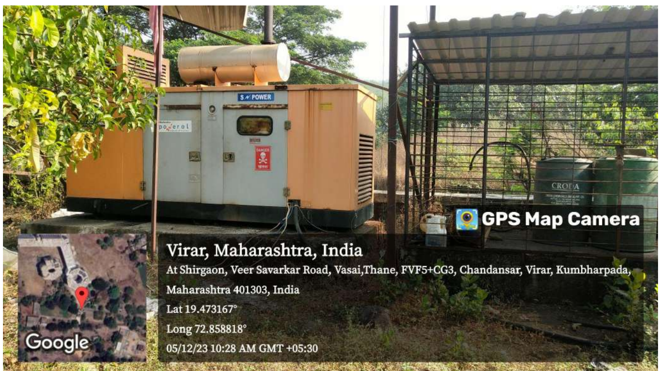
Generator in campus
